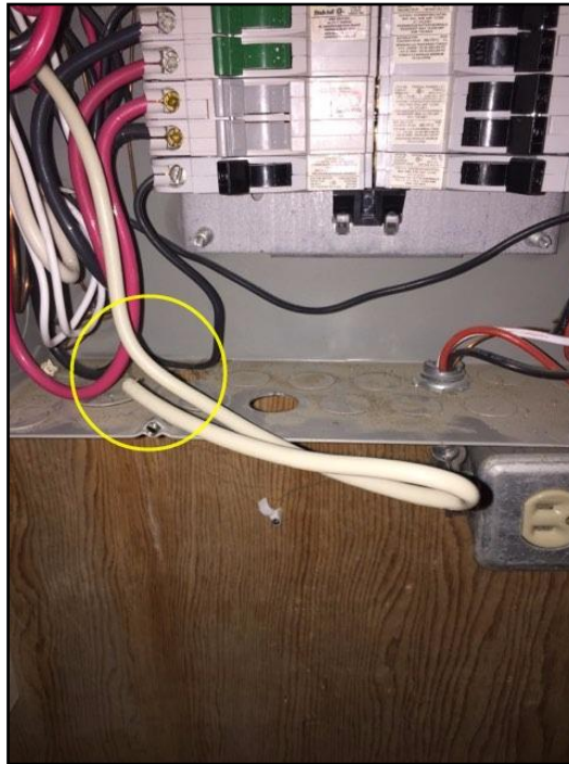
39. Abandoned wires in panel
