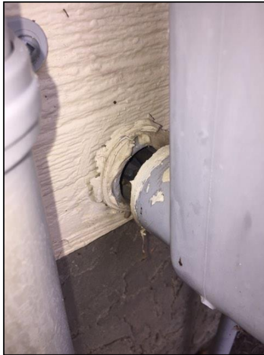
38. Conduit or cable damaged
