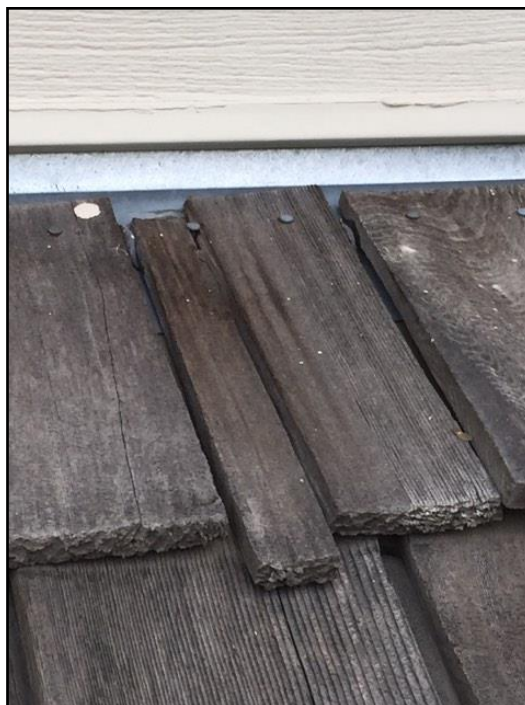
5. Damaged, broken or missing pieces
