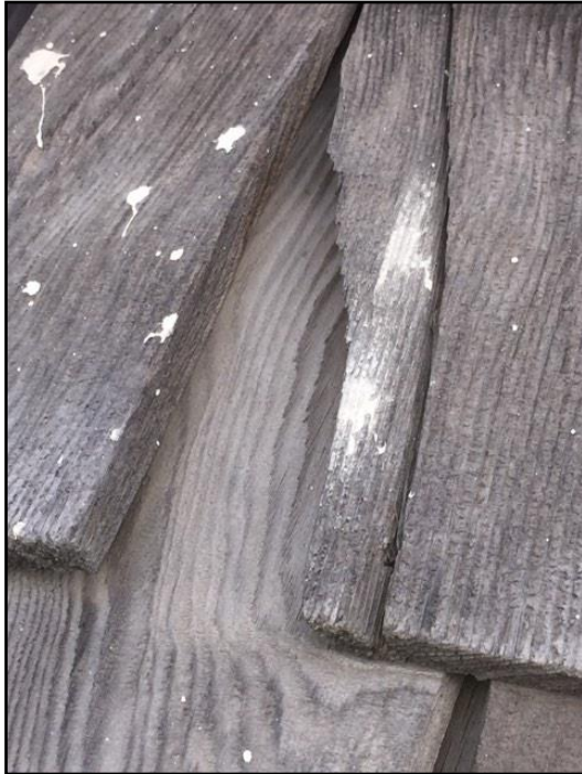
3. Damaged, broken or missing pieces
