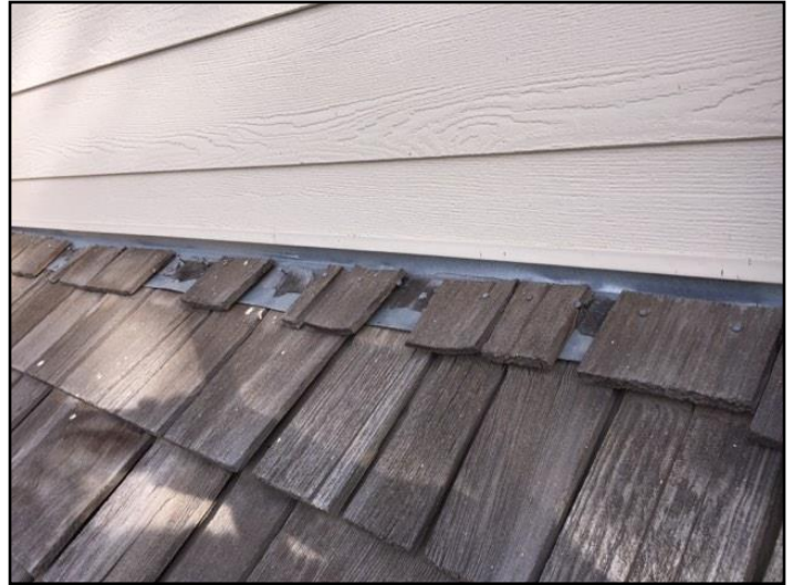
4. Damaged, broken or missing pieces
